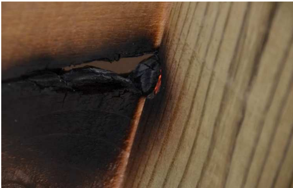
Figure 3. Detail of the underside of the decking assembly (cedar). The ignition process was observed to spread to the wood supporting members [10].
