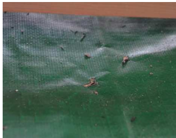
Figure 6. Images of Sarking Placed Under Concrete Tiles (profiled tile) Taken Immediately after the Experiment was Completed. The Tiles have been removed [12].
