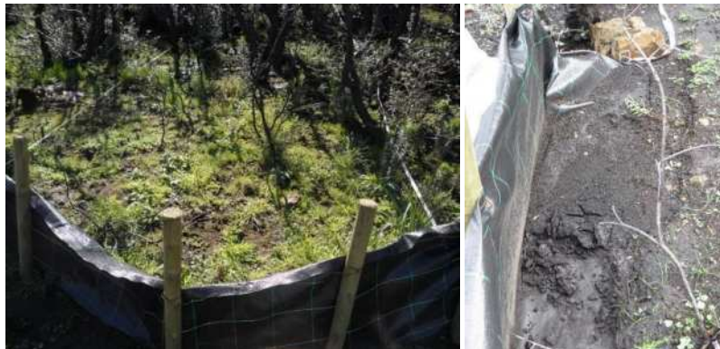
Figure 2. Example of sample plot and sediment trapped in the silt fence
